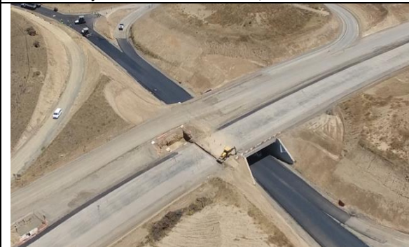
Vista general – P.S. Campiche Sector 2.
